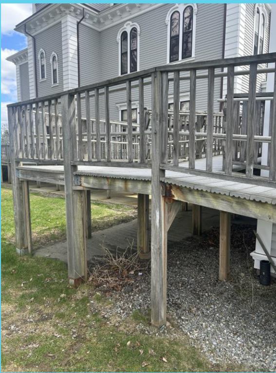
Ramp to upper level of first floor is non-compliant and in disrepair
