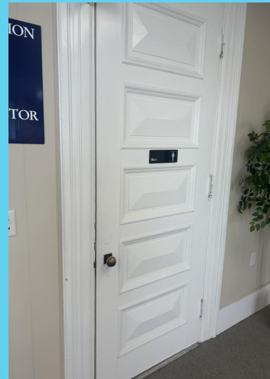
No accessible bathrooms, door hardware or, service windows
